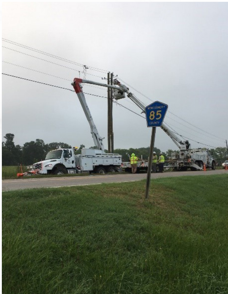
An Alabama Power crew replaces a power pole that was struck by a vehicle and caused 166 customers to lose power for six hours in Montgomery, Alabama.
