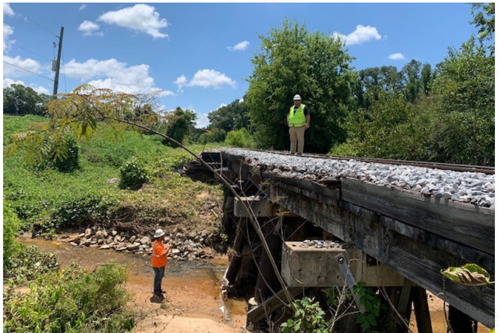
Chris Hester, Railway Safety Administrator, supervises Heath Thompson, Rail Safety Track Inspector, as he inspects underneath a railroad bridge for a closer look at an alignment issue on the ballast retainer.
